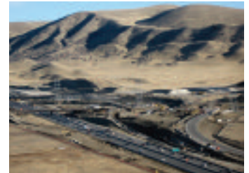
A new interchange is under construction along C-470, south of I-70, where beltway construction first began in 1980.
